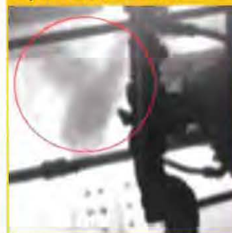
Leaking Valve as shown by Infrared Camera
