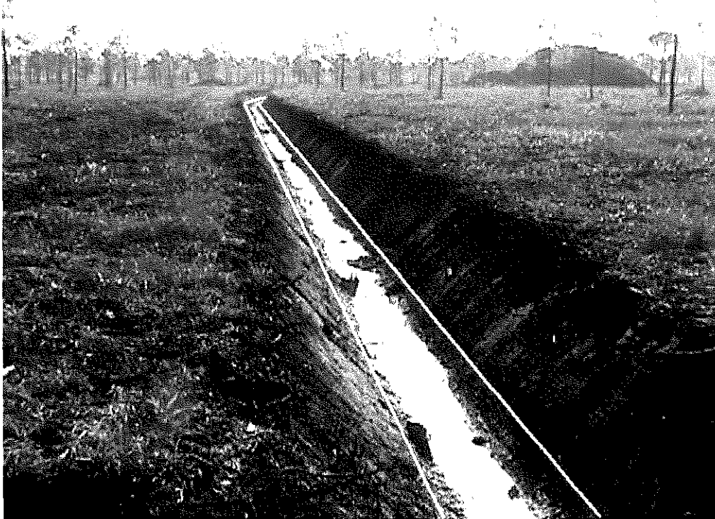
Photo 53. Drainage ditch, an RPW, South Atlantic Division. Ditch excavated in wetlands; ditch is subject to jurisdiction under CWA. Yellow lines mark approximate location of OHWM.
