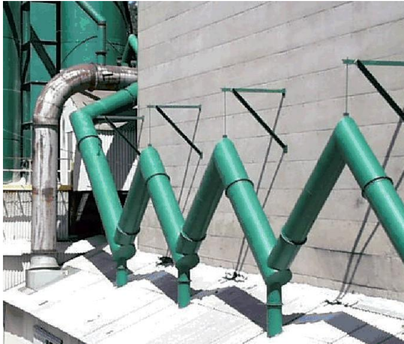
Figure 1.10. Sawtooth design of a low-velocity system with a dropout duct back into the process at the base of each leg.
