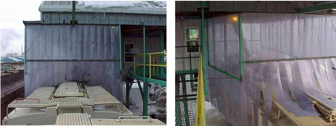
Figure 7.7. Rail car loadout area enclosed with plastic strips to contain dust.
