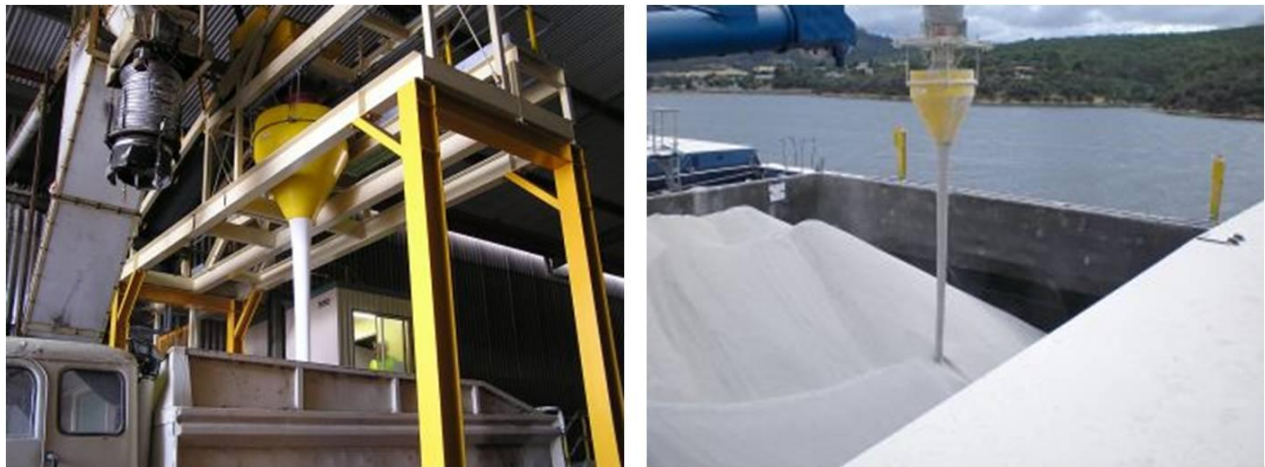
Figure 7.6. Dust Suppression Hopper creating a solid stream of material during loading to reduce dust liberation.
