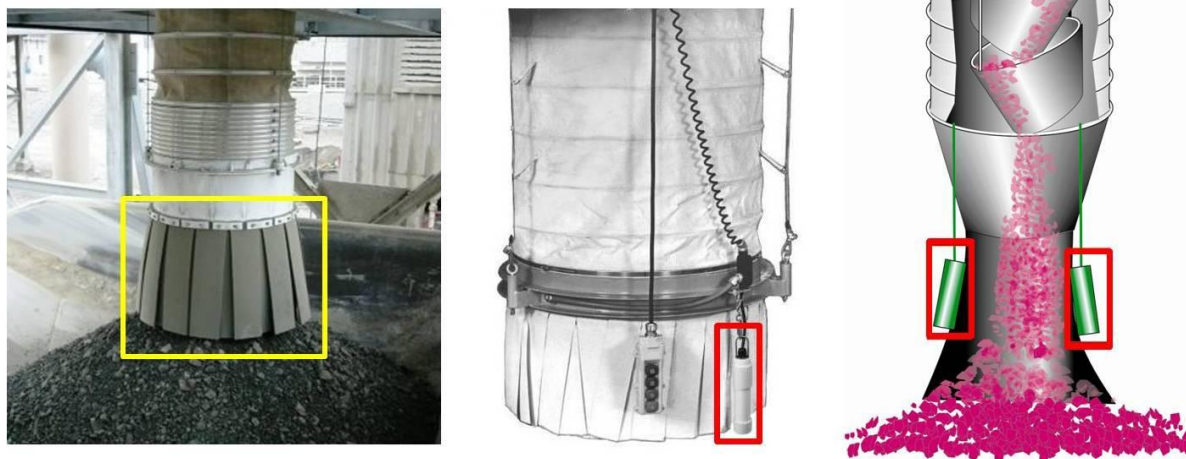
Figure 7.4. Skirt (in yellow box) and tilt sensors (in red boxes) installed on the discharge end of loading spouts to help reduce dust emissions.
