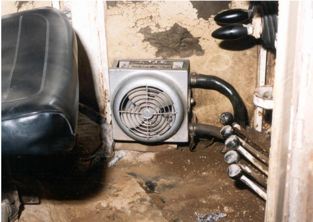
Figure 8.13. Product tracked onto the floor of a piece of mobile equipment from dirty work boots.
