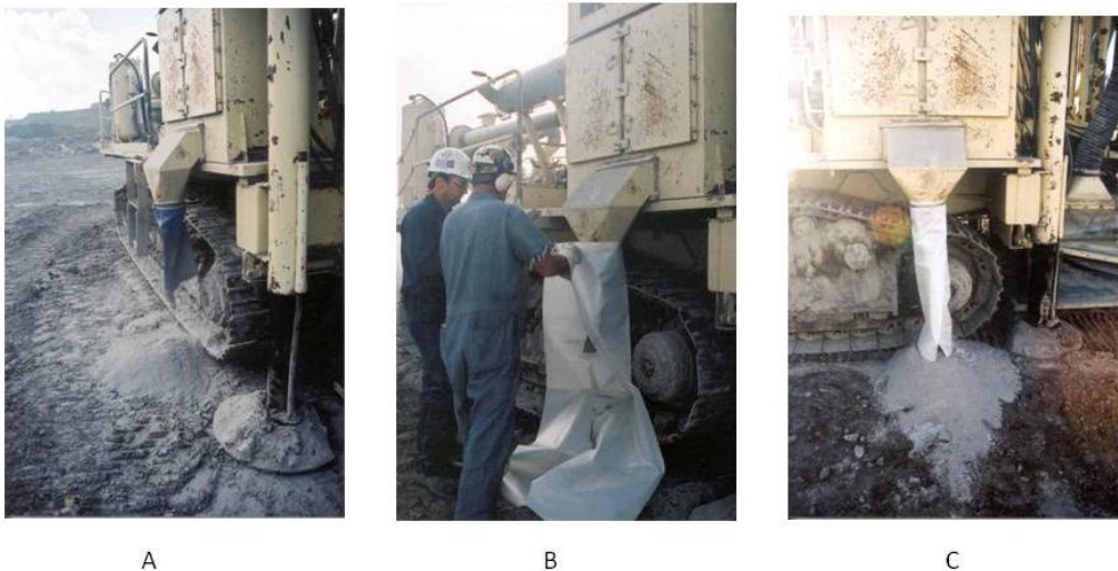
Figure 3.13. Dust collector dump point prior to shroud installation (A). Two men installing the shroud onto the dust collector dump point (B). The dust collector dump point after installation of the shroud (C).
