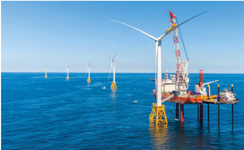
Installation of Deepwater Wind's Block Island Wind Farm, off Rhode Island. While offshore wind energy projects have not yet been developed in the Mid-Atlantic, several areas have been leased for that purpose. © DEEPWATER WIND
