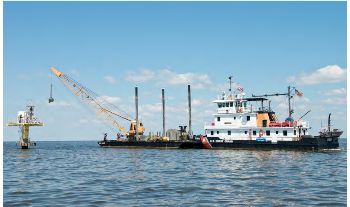
Crewmembers aboard Coast Guard Cutter Sledge use the ship's crane to lower a new transformer down to Craighill Entrance front range light Aug. 25, 2014. Crew members from Aids to Navigation Team Baltimore help guide the transformer onto the structure by use of the tag line.
